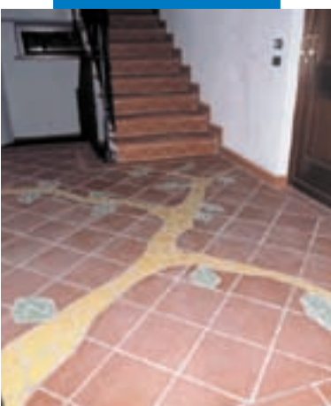
An example of a floor in terracotta tiles and porcelain inlays treated with Keraseal - Mozzata (Como) - Italy
