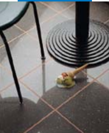
An example of a grout in a public premises
